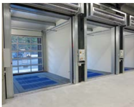
Integrated into the loadhouse
